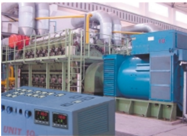
Typical Application – Power Generation
