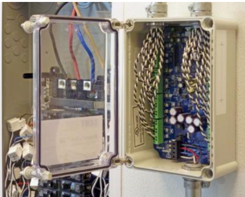
Power Squad mounted in a NEMA-rated box near electrical panel
